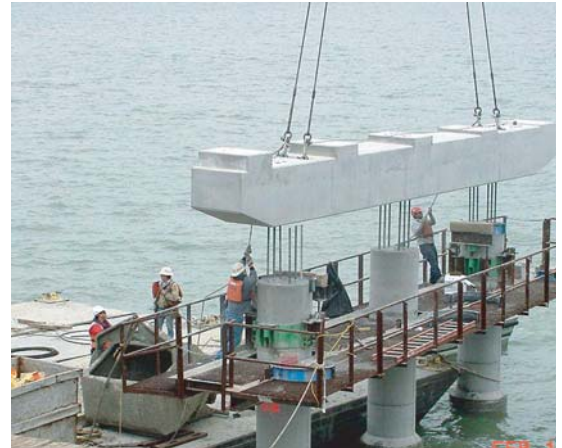
Precast bent cap being placed into position, SH 66 bridge over Lake Ray Hubbard.
