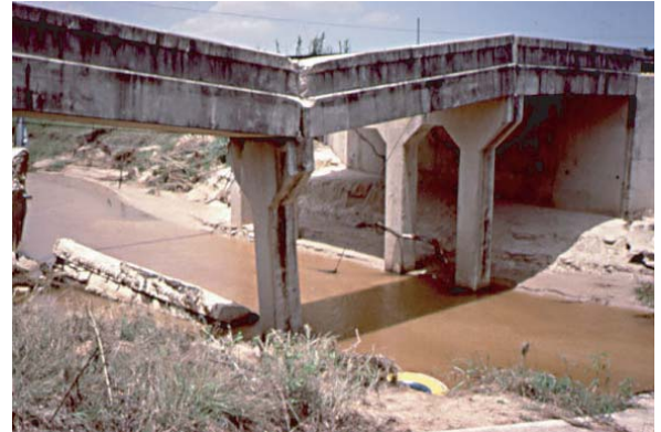
Scour of soil from around bridge piers can ultimately lead to structural failure
