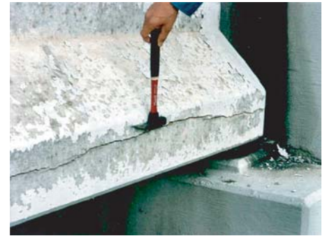
Prestressed concrete beam with Premature Concrete Deterioration
