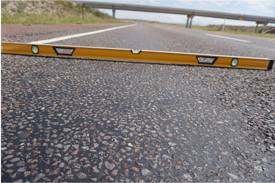
Figure 65. Pavement Surface Rutting on I-10.
