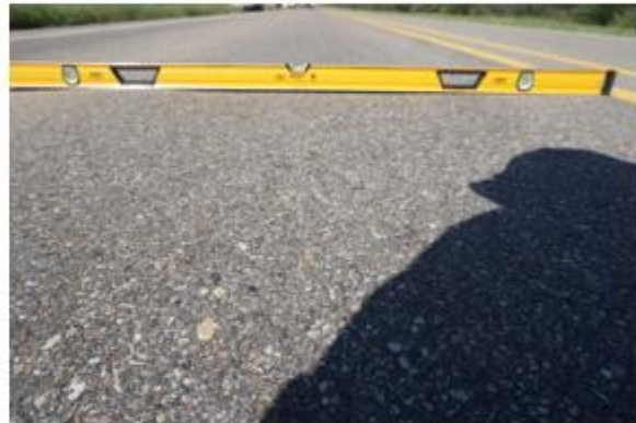
Rutting in Inner Wheel Path: 1/16–8/16 in. 10/09/2017
