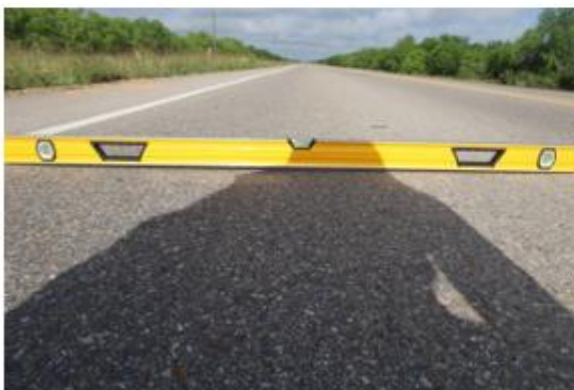
Rutting in Outer Wheel Path: 1/16–8/16 in. 03/29/2018
