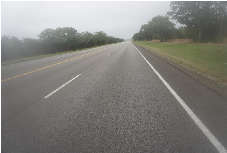
Figure 72. No Cracking on the Test Section with PG70-28 on SH 71.
