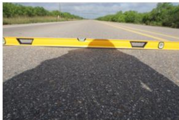
Rutting in Inner Wheel Path: 1/16–8/16 in. 03/29/2018
