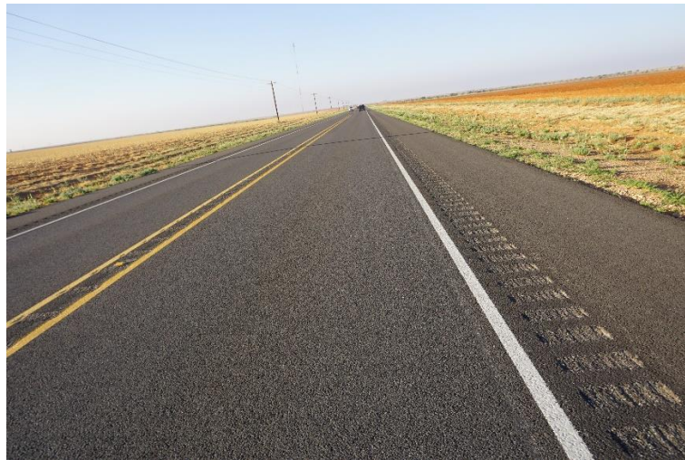
Figure 54. No Cracking on the Test Section with PG70-28 on SH 214.
