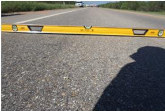
Rutting in Outer Wheel Path: 1/16–8/16 in. 10/09/2017
