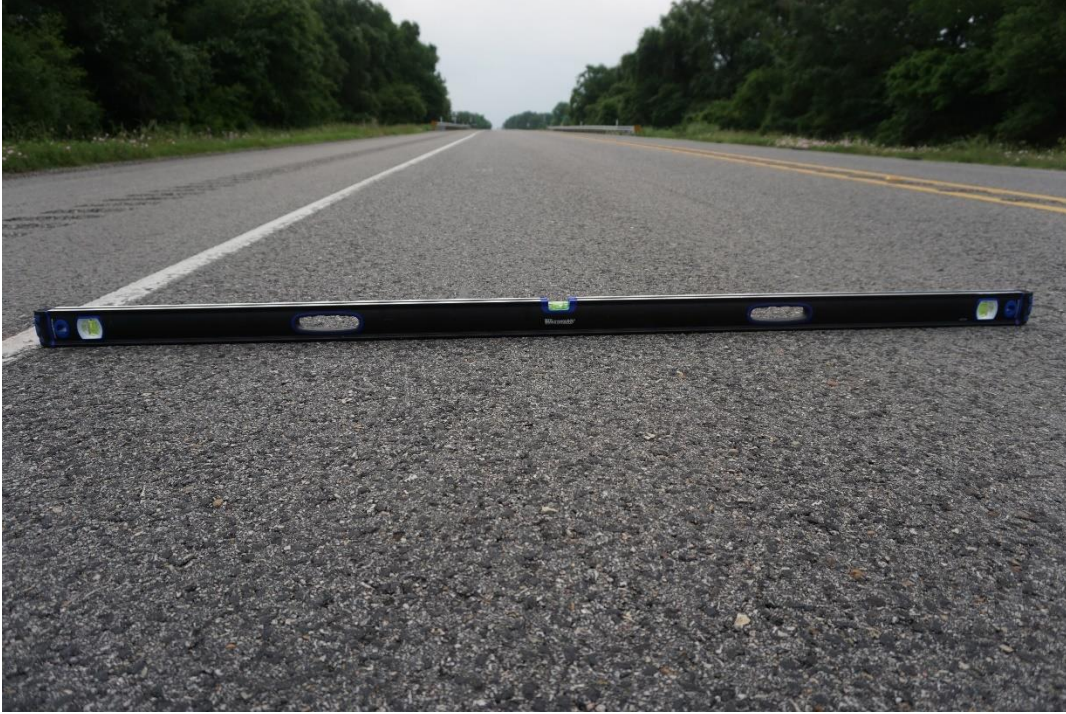
Figure 42. No Rutting on Both Test Sections on SH 7.
