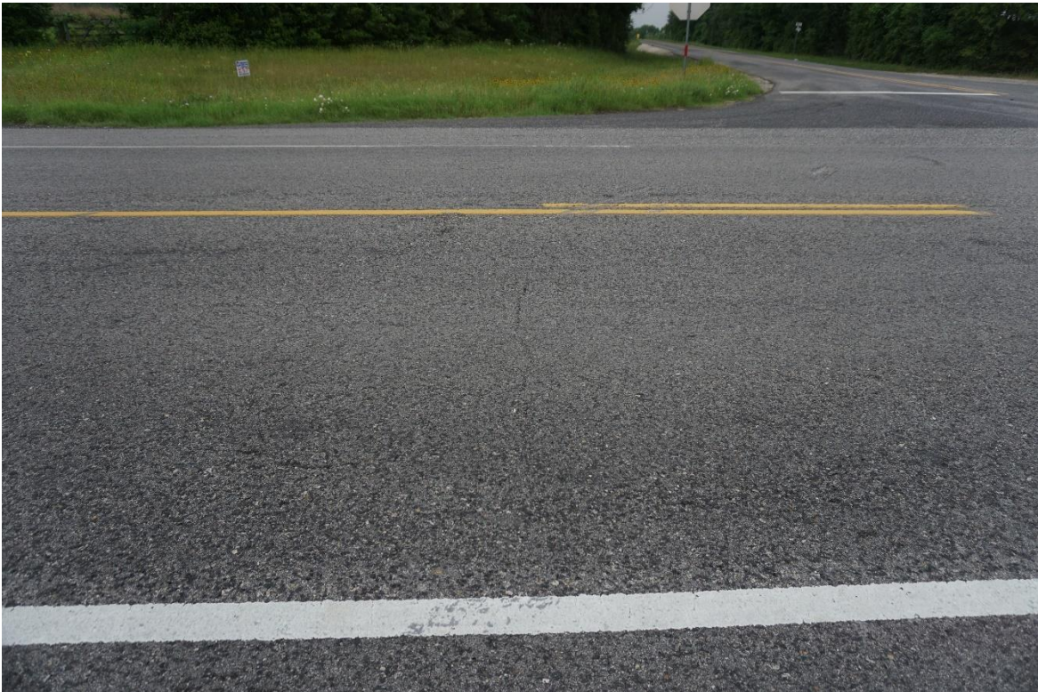
Figure 43. Cracking Observed on Control Section with PG64-22.
