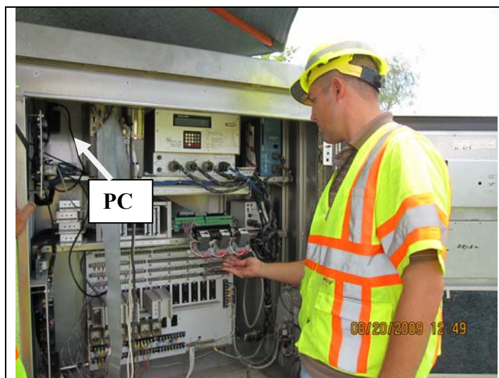
Figure 6. Equipment Installed in Caldwell Controller Cabinet.
