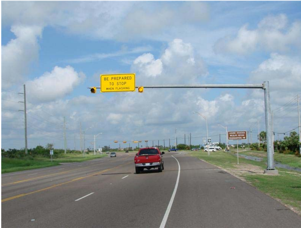
Figure 6. AWECS Installation in Pharr District.
