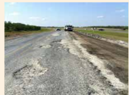
Figure 2. Major Damage Requiring Rehabilitation.
