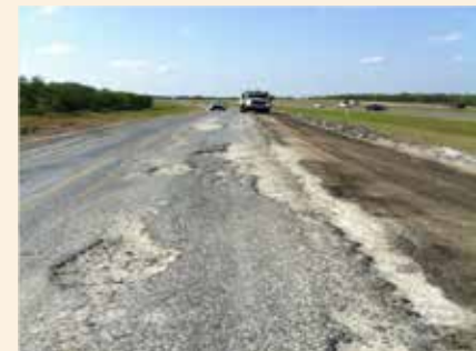
Figure 2. Major Damage Requiring Rehabilitation.
