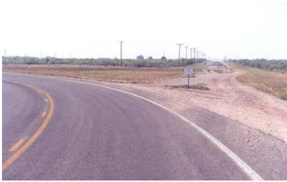
Figure 7-7. Obliterated Roadway Section.
