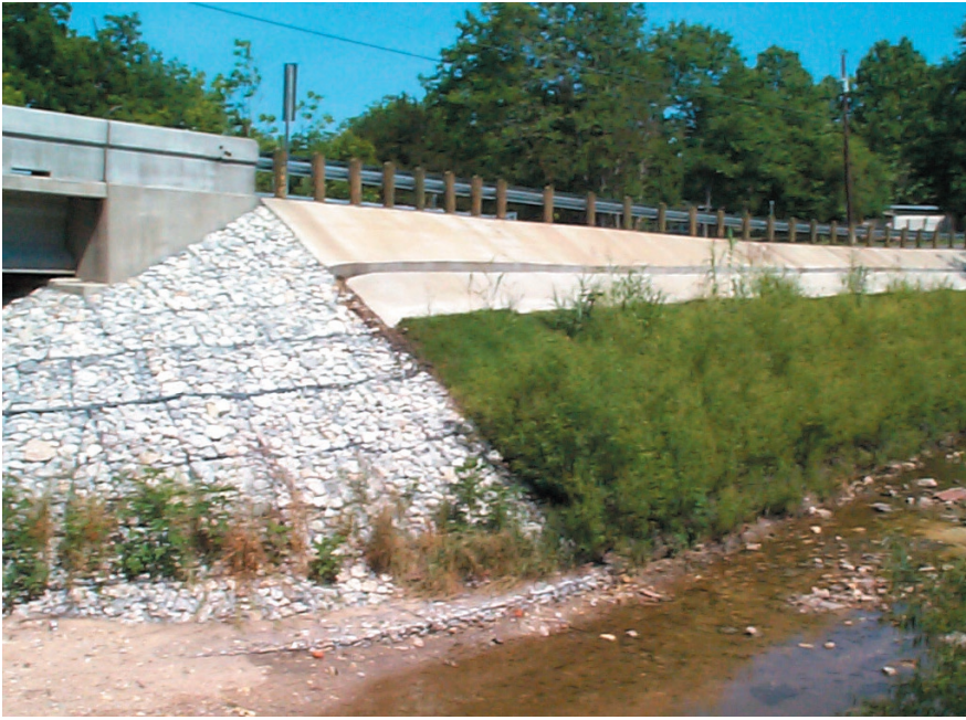
Figure 2. Gabion mattress abutment and streambank stabilized by vegetated geogrids. (Photo taken in May 2002)
