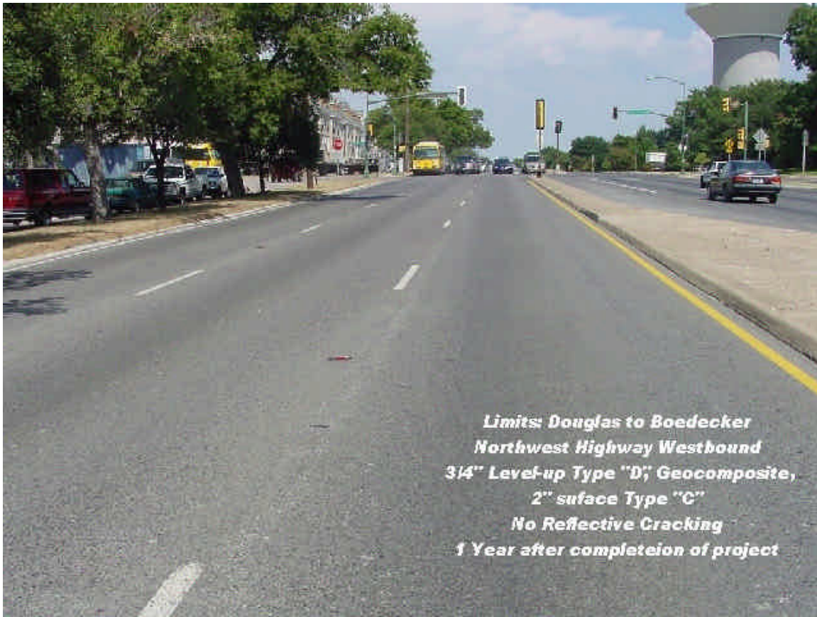
Figure D6. Westbound Direction of Loop 12 after One Year of Service.
