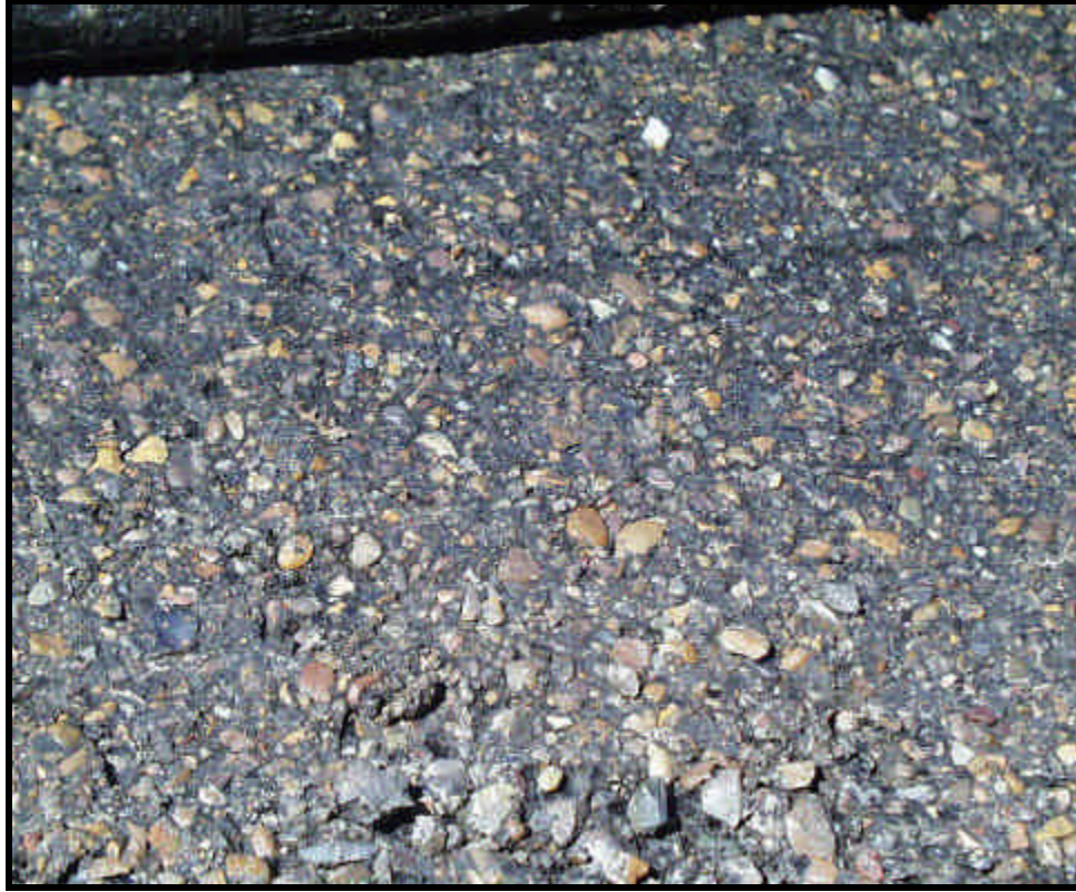
Figure D11. Stripping of Underlying Type B HMA Layer. (Note indentions from geocomposite material.)
