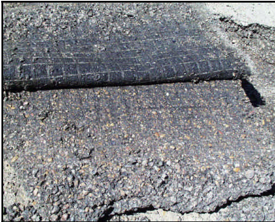
Figure D10. Geocomposite Material Delaminating from Lower Type B HMA Layer.
