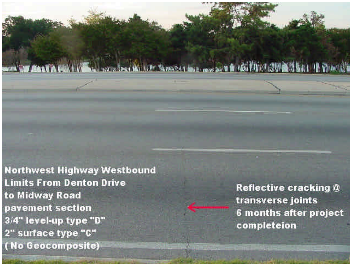
Figure D7. Transverse Cracking with a Level-up Course and Without Geocomposite.
