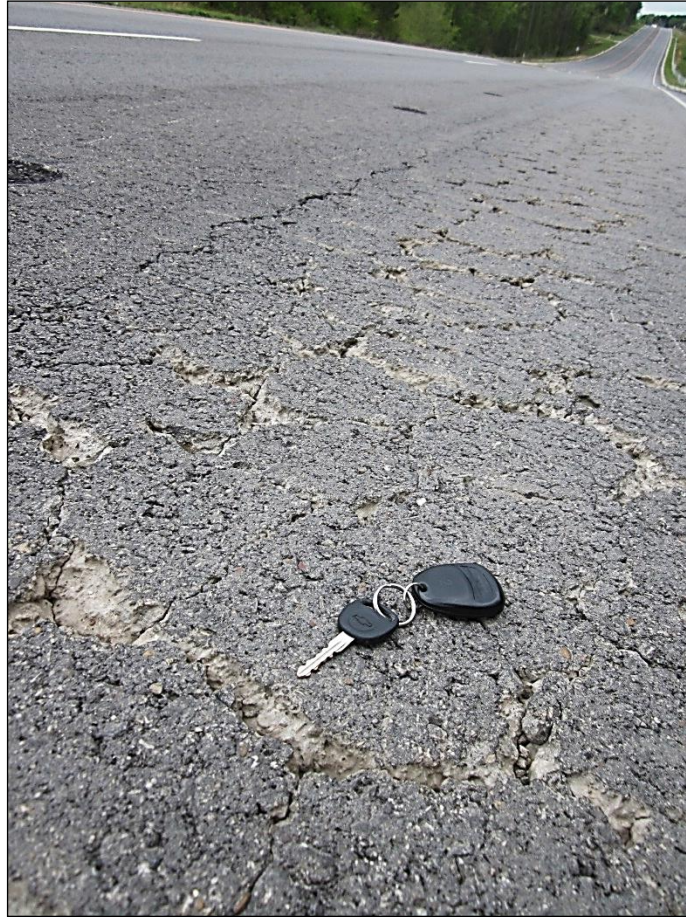
Figure 60. Premature Fatigue Cracking, Project 3.
