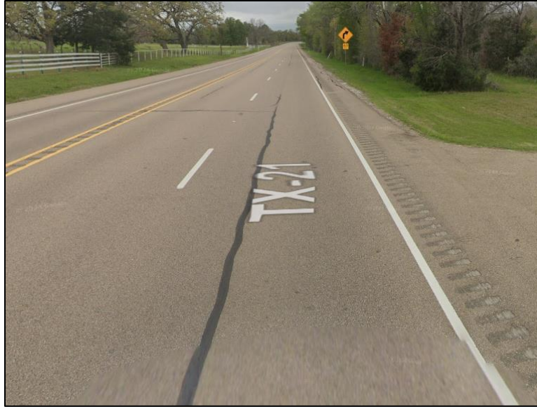
Figure 2. Longitudinal Crack in a Widened Pavement.
