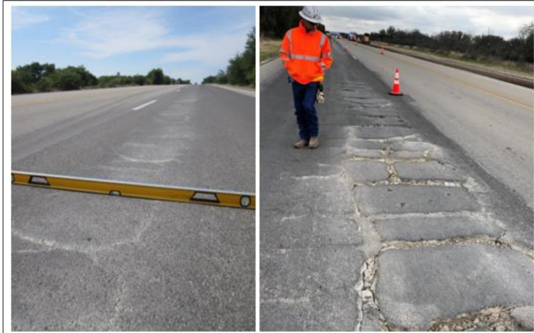
Figure 8. Failure of US 83 on Inside Lane.
