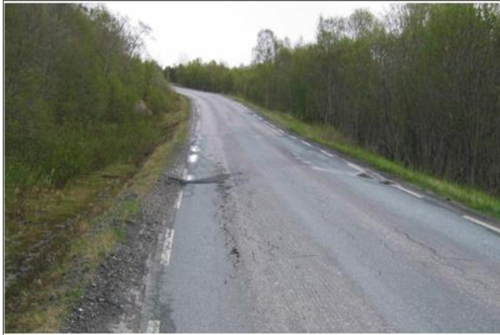
Figure 11. Edge and Drainage Failure (6).
