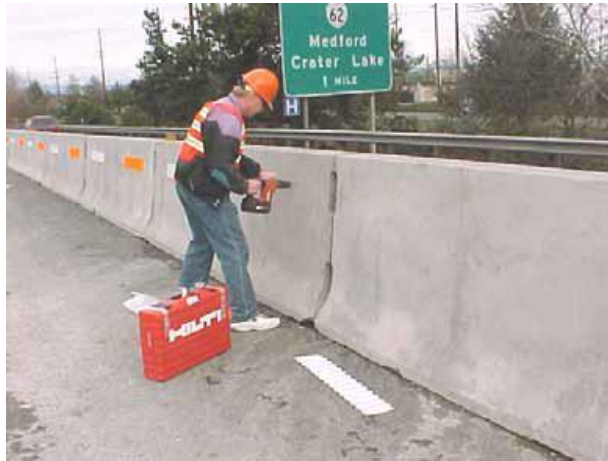
Figure 10. Typical LDS Panel Installation in Oregon (4).
