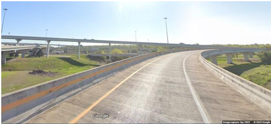
(b) Street view of the treated ramp from I-20 EB to I-35W SB
