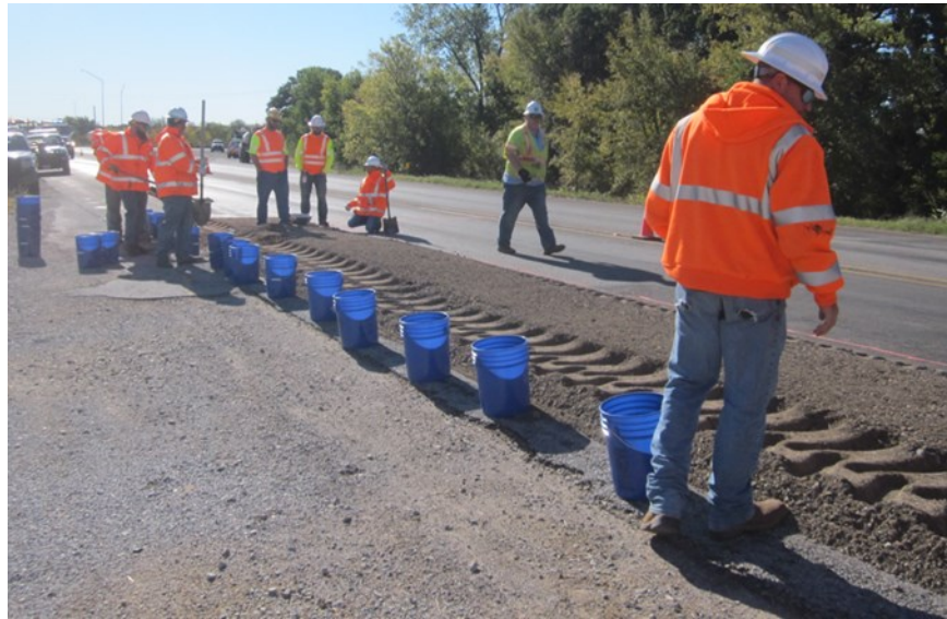
Figure 42. ILS materials sampled from the roadway BWD FM 2214.
