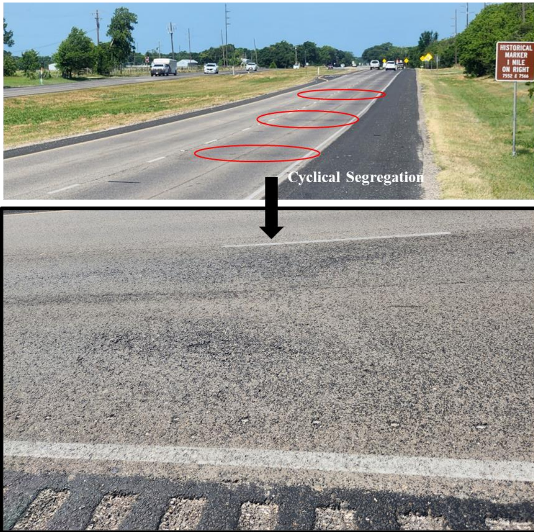
Figure 111. Cyclical Segregation on RMC Project.
