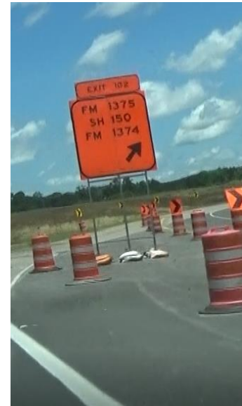
(c) Exit direction sign
