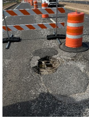
(h) Development of a hole on deck (WFS-RC-07)
