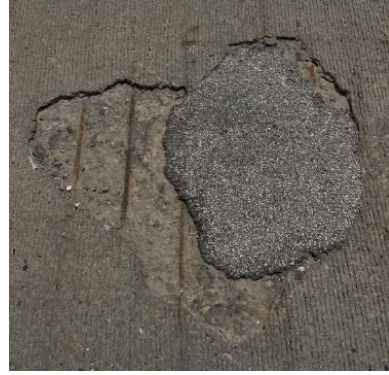
(b) Exposed Rebar on Deck due to Delamination
