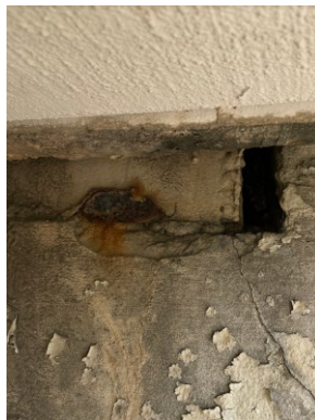
Figure 0.266. Corrosion near Bearing Pad
