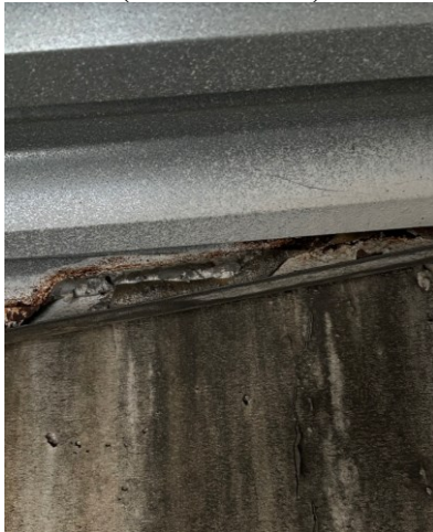
(e) Corrosion detected at deck (FTW-RC-04)
