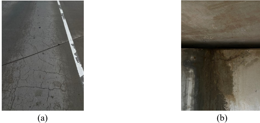
Figure 0.193. Deterioration on the Bridge: (a) Map Cracks Propagating from a Joint; (b) Cracks and Leakage at Abutment
