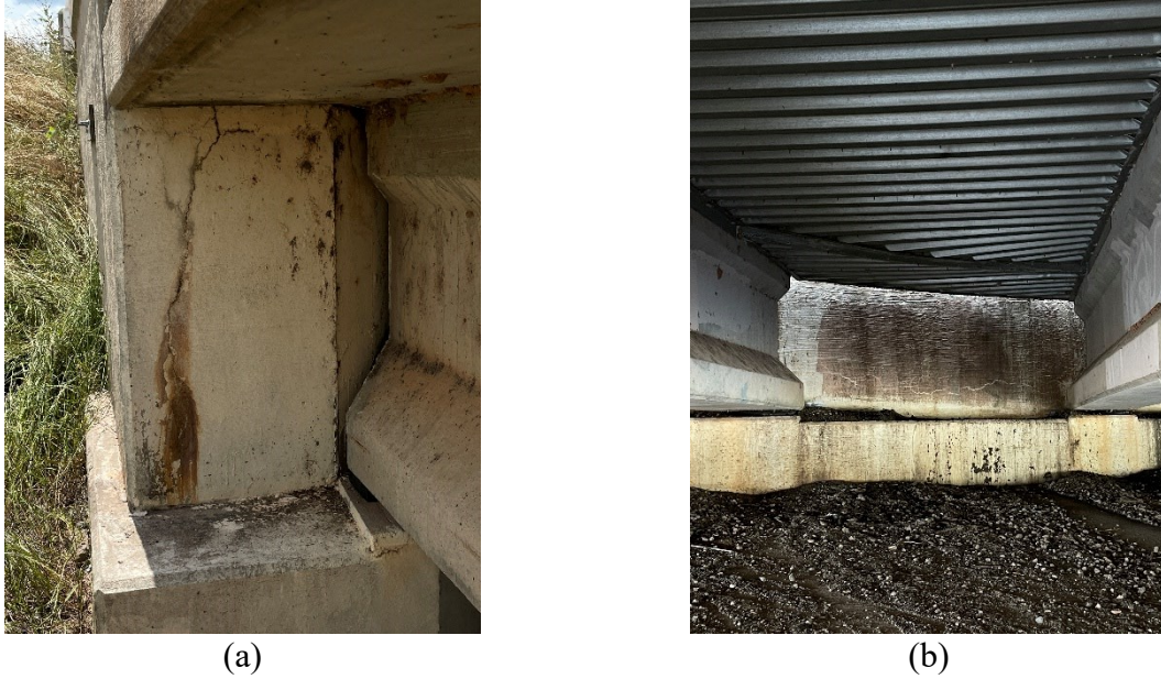
Figure 0.403. Deteriorations on the Bridge: (a) Vertical Crack and Efflorescence at Abutment Wall; (b) Horizontal Crack and Efflorescence at Abutment Wall
