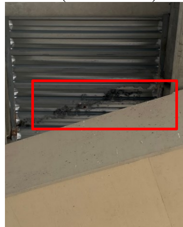
(f) Corroded metal deck form near joint (WFS-RC-04)
