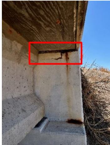
(c) Cracks at abutment backwall (CHS-RC-06)
