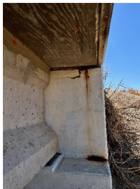
Figure 0.185. Deteriorations on the Bridge: (a) Cracks at Abutment Backwall
