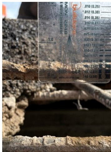
(i) Pitting corrosion where the hole was (WFS-RC-07)
