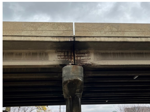
(b) Spalling at Girder End Due to Corrosion
