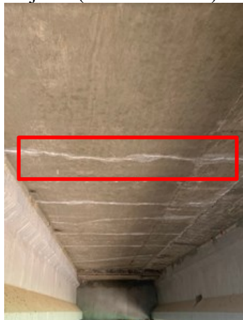
(e) Cracks and efflorescence on bottom surface of deck (AMA-RC-08)
