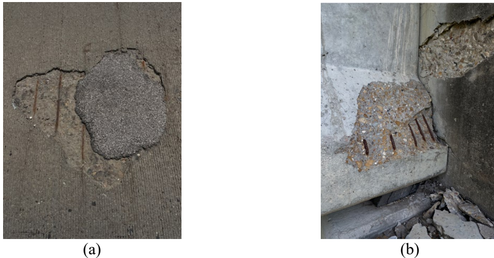
Figure 0.339. Deteriorations on the Bridge: (a) spalling on deck; (b) Exposed rebar on the girder end
