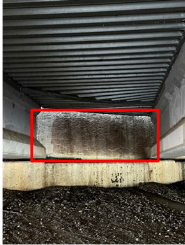
(g) Horizontal cracks and efflorescence at abutment backwall (WFS-RC-05)
