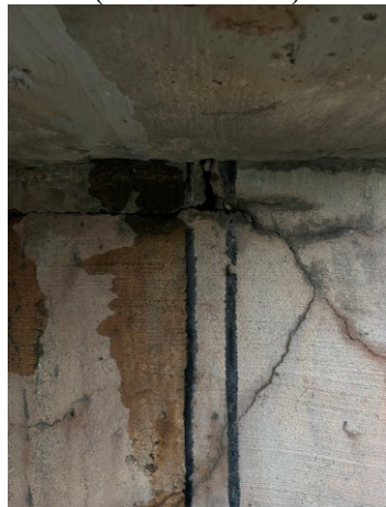
(e) Crack at abutment backwall (WFS-RC-03)
