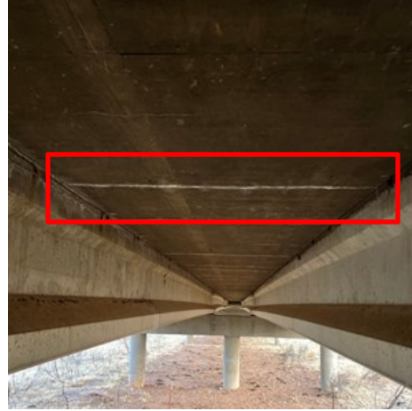
(b) Moderate cracks on bottom surface of deck (CHS-RC-05)
