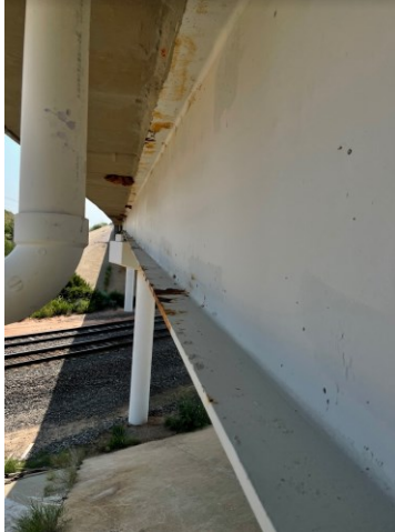
Figure 0.310. Pitting Corrosion on the Web and Bottom Flange
