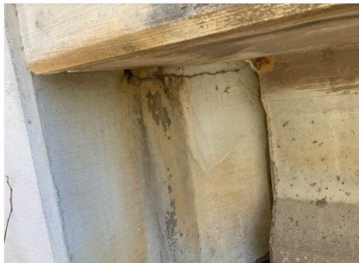
Figure 0.281. Crack and Efflorescence at the Abutment Wall
