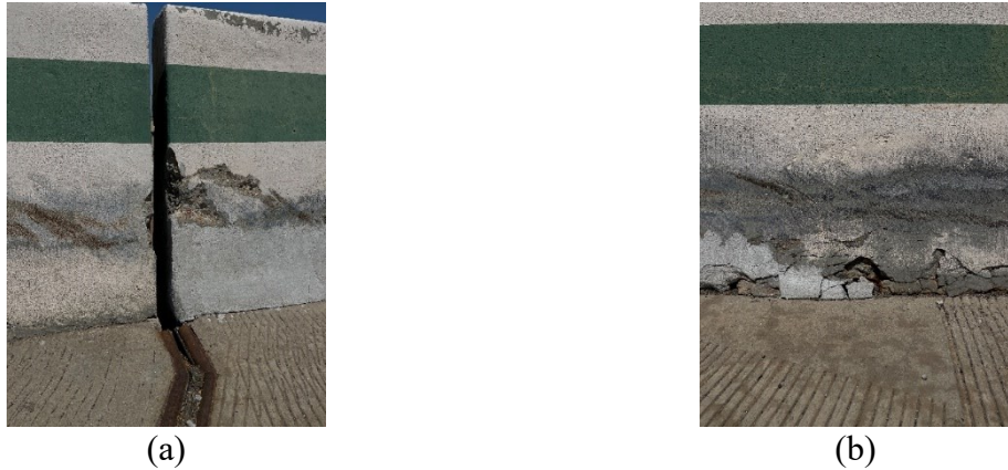
Figure 0.43. Deterioration on the Bridge: (a) Impact Damage on the East Rail of the Bridge; (b) Exposed and Corroded Rebar
