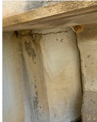
(f) Crack and efflorescence at abutment backwall (FTW-RC-05)
