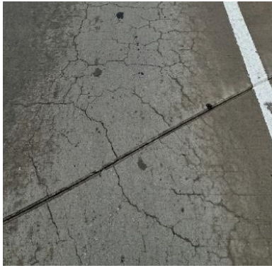
(a) Cracks at Deck Joint
