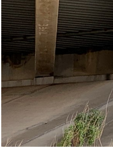
(c) Corrosion at metal deck from an abutment (ELP-RC-06)
