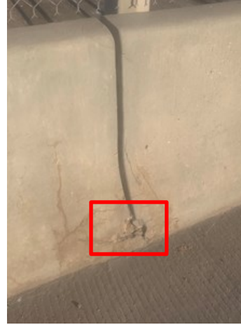
(b) Rust at rail bottom (AMA-RC-04)
