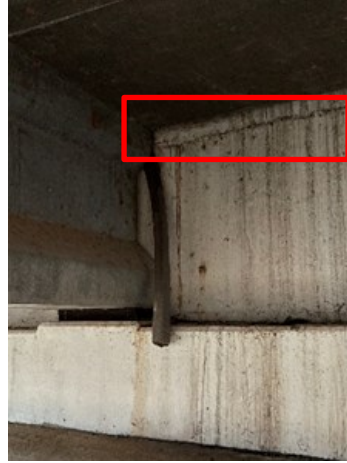
(m) Hairline cracks at abutment back wall (CHS-RC-04)
