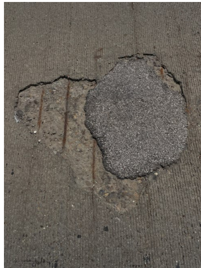
(b) Exposed Rebar on Deck (LBB-RC-04)
