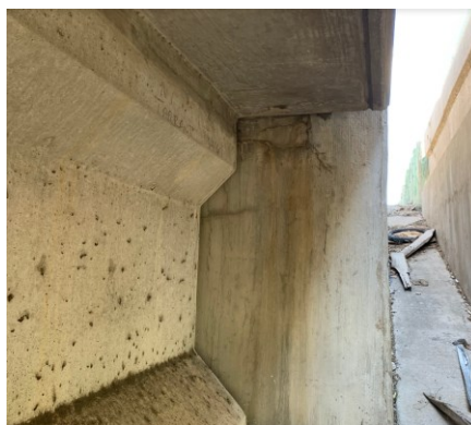
Figure 0.289. Cracks at Abutment Wall
