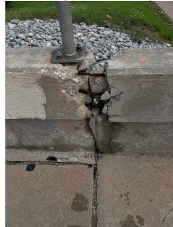
(d) Exposed and corroded rebar at concrete rail (WFS-RC-03)
