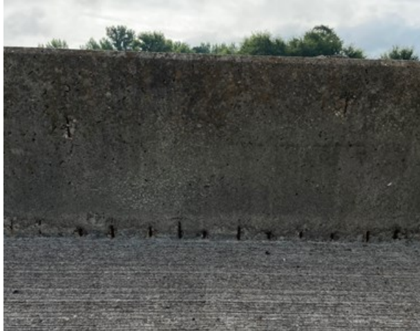
Figure 3.16. Exposed and Corroded Rebar at Concrete Rail at ATL–RC–01 in Region 4.
