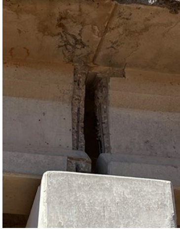
(g) Spalling and exposed rebar at girder ends (CHS-RC-01)
