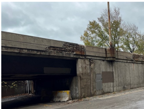
(a) Spalling at Rail Due to Corrosion
