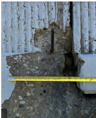
(g) Exposed and corroded rebar at abutment (TYL-RC-02) Figure 3.15. Deterioration of Bridges in Region 3 (Cont.).
