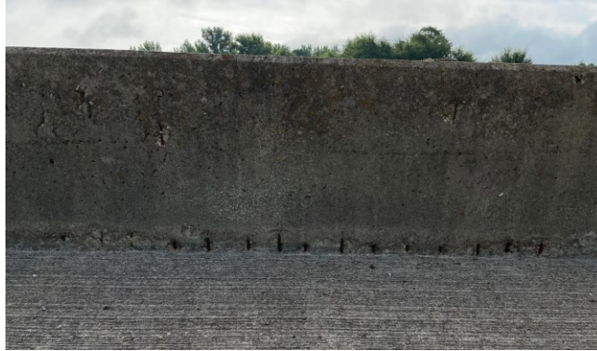
Figure 0.93. Exposed and Corroded Rebar at the Bottom of Railing
