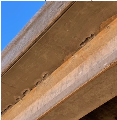
(k) Concrete fall-off at intersection of replaced overhang (CHS-RC-01)
