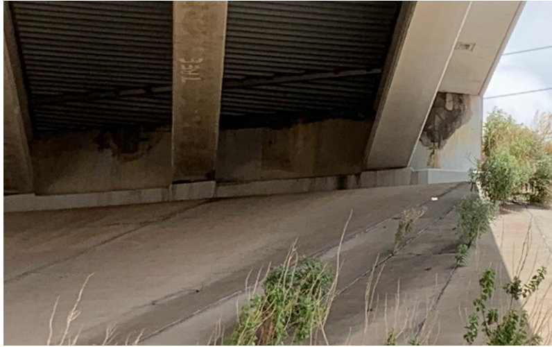
Figure 0.229. Corrosion at metal deck form and abutment
