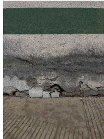
(d) Exposed rebar due to impact damage on a rail (AMA-RC-06)
