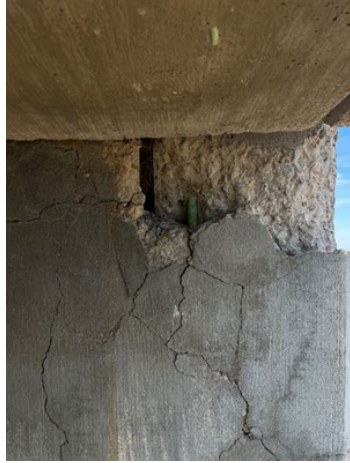
(a) Exposed and corroded ECR due to spalling at abutment (AMA-RC-02)
