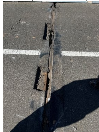
(f) Spalling of overlay at joint (CHS-RC-01)
