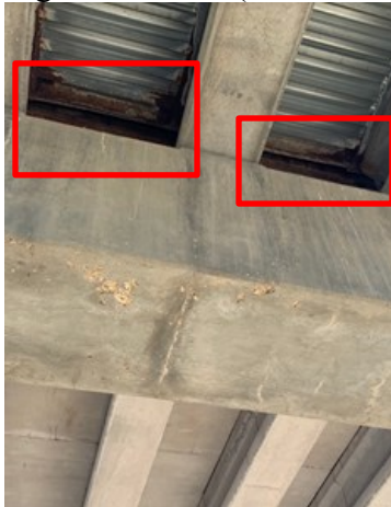
(c) Corrosion on the metal deck form near a joint (AMA-RC-04)
