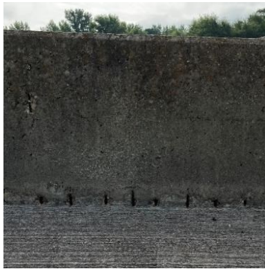
(c) Exposed Rebar on Concrete Rail
