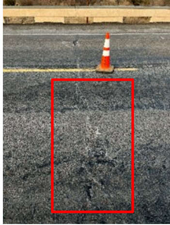
(a) Cracks and delamination of asphalt overlay (CHS-RC-05)
