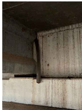
Figure 0.169. Deteriorations on the Bridge: Hairline Cracks on Abutment
