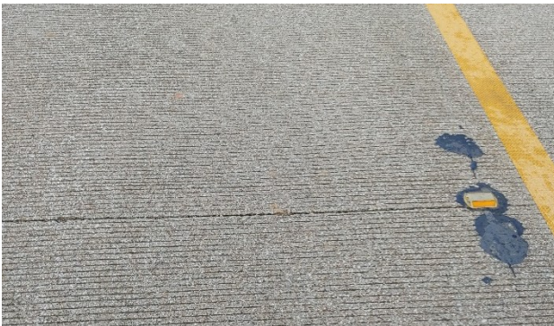
(c) Main PBJ crack
