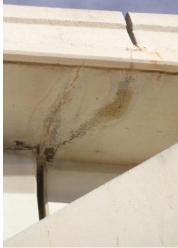
(b) Cracking on bottom of overhang
