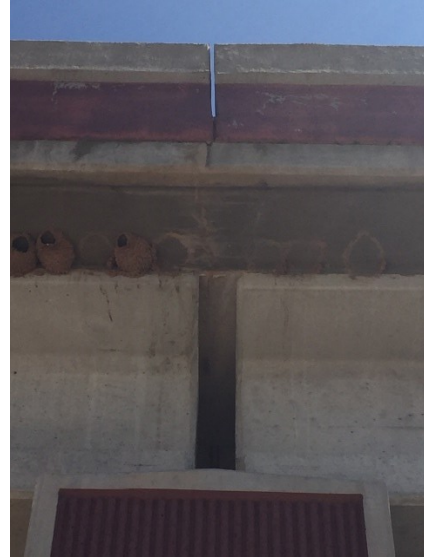
(b) Cracking and efflorescence in overhang
