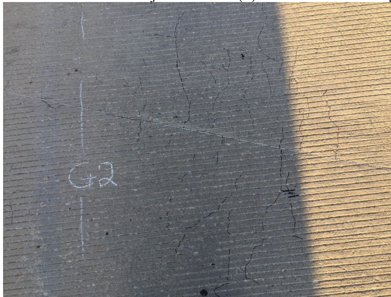
(c) Marked cracks in NDE region
