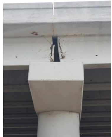
(c) Girder end damage
