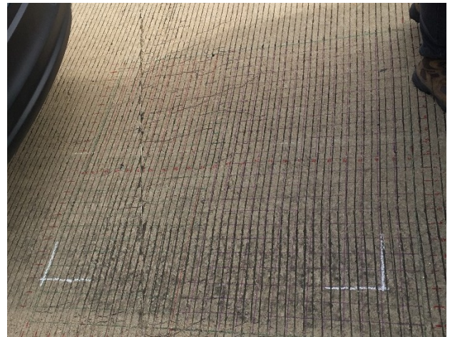
(b) Cracks in NDE region
