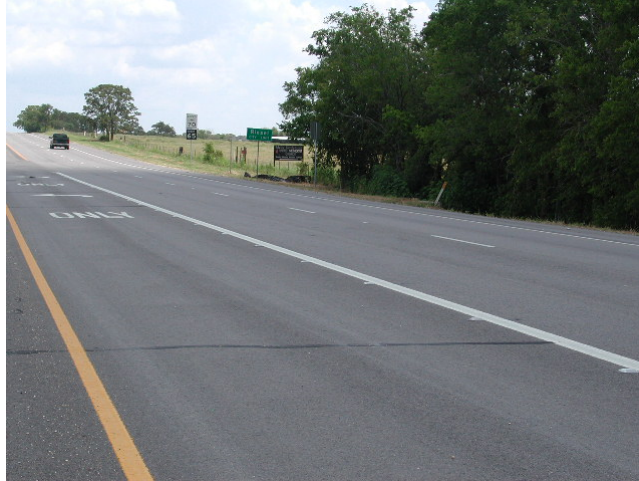
Figure 12. Reflection Cracking on the Left Lane of SH6.
