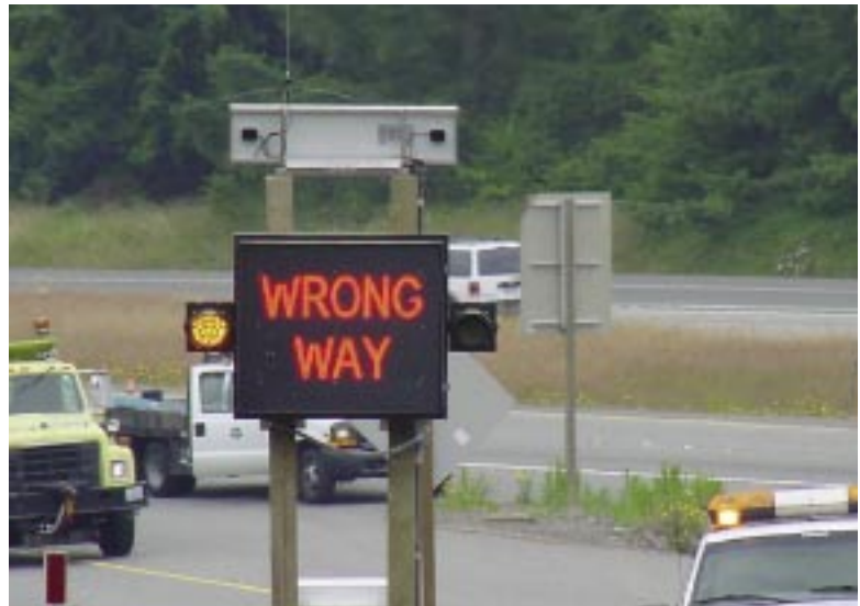
Several states use ITS applications like this changeable message sign to deter wrong-way movements.
