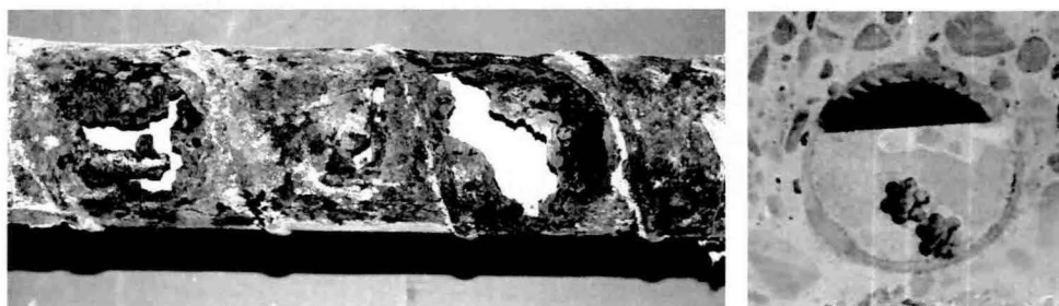
Figure 3.16 Bleed Water Void and Duct Corrosion
