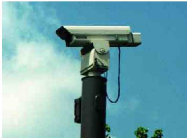
Figure 1. TMC Closed-Circuit Television Camera for Visual Traffic Information
