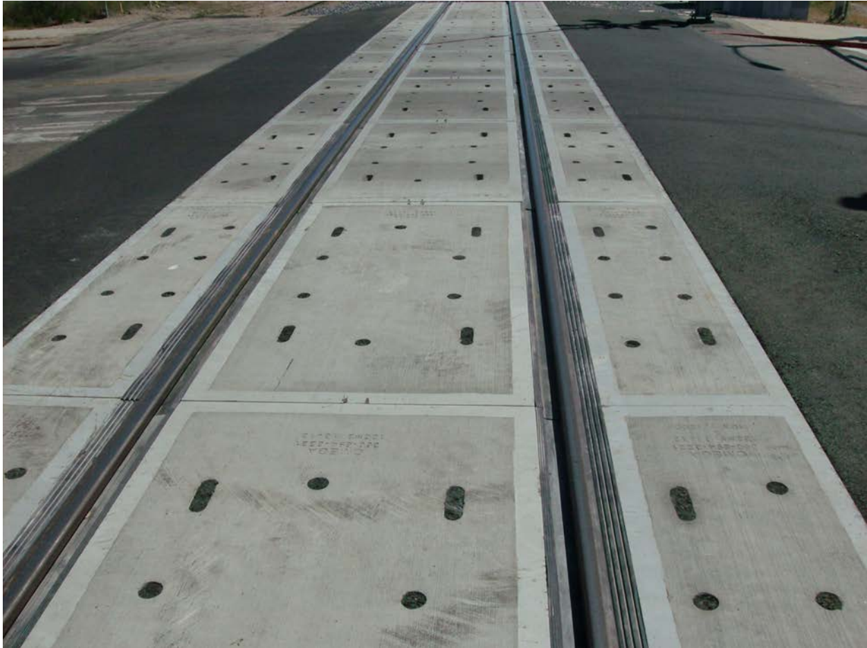
Figure 10. Recently Completed Metrolink Osborne Street Crossing on the Antelope Valley Line in the Sun Valley Area of Los Angeles.
