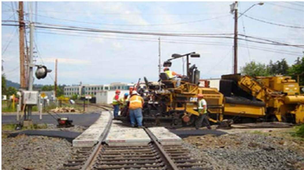
Figure 9. WES Commuter Line Crossing (SW Durham Road) on Portland & Western RR near Portland, OR, one of 13 Crossings Underlain with Asphalt.
