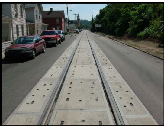
Figure 2c. NS Crossing in West Brownsville, PA, the 3226-ft (983-m) long Crossing is being Replaced in Segments over four years.
