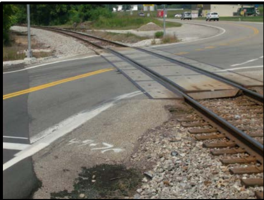
Figure 2a. CSX Crossing on WV Route 2 at Ashton, WV, Perfect Condition after 11 years.
